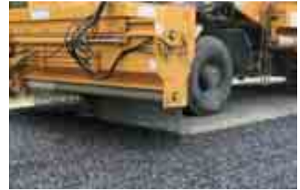
Smaller, top stone, spread at 24 to 25 lb per sq yd, will interlock with bottom stone when compacted by rollers.
