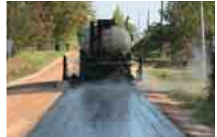
Charles E. Watts, Inc.'s E.D. Etnyre & Co. distributor sprays high-float emulsion at rate of 0.395 gal per sq yd on Route 29 surface following reclamation by Cherokee County, Ala., forces.
