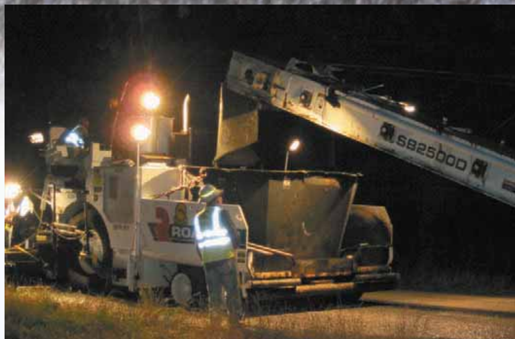
Contractor employs a ROADTEC SB-2500D shuttle buggy to feed material to a ROADTEC RP-190 spreader paving machine.
