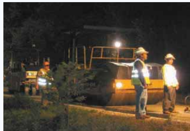
Three CAT rollers compact mix: a CB634D vibratory roller, a PS150C pneumatic roller, and a CB534D static roller.
