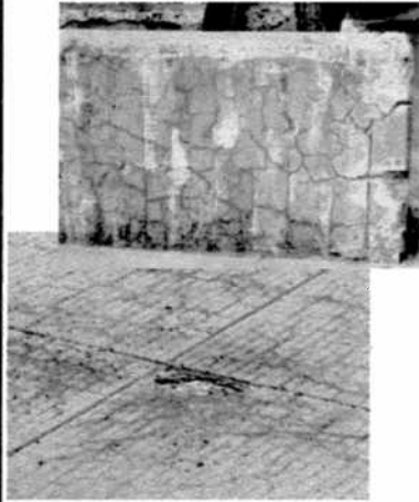
ASR-affected concrete wall (above) and joint damage on an ASR- affected pavement (below).
