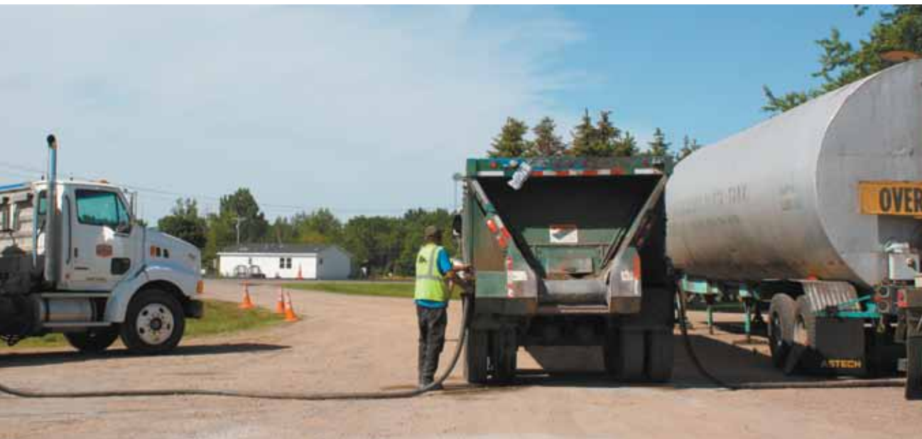
A ‘nurse’ truck takes on a load of emulsified HiMA binder with a grade of CSS1-h supplied by Flint Hills Resources.
