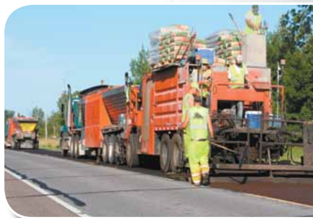
ASTECH Corporation applies micro surfacing containing emulsified highly polymer modified asphalt to a section of Trunk Highway 23 for Minnesota DOT.
