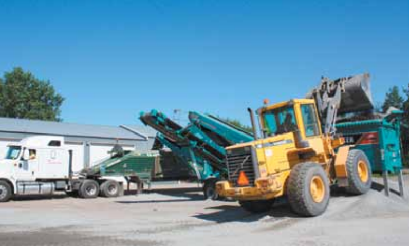
A Volvo L70D fills hopper of a Terex Powerscreen Chieftain 600 which processes aggregate used to make micro surfacing mix.
