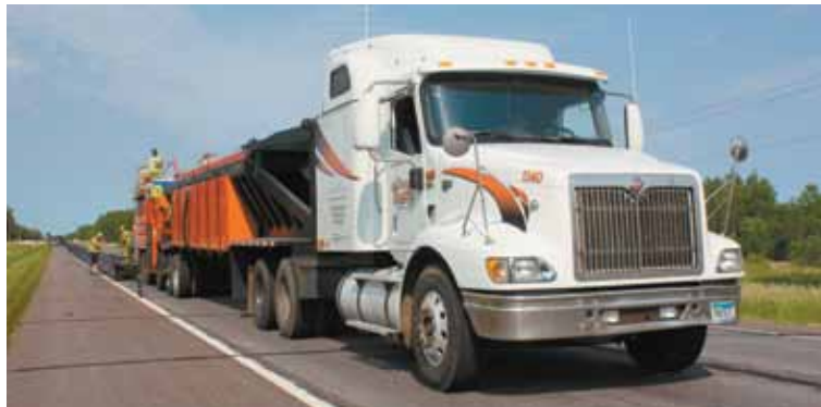
An International nurse truck leads micro surfacing train on TH23, a road that experiences an average daily traffic count of more than 5000.
