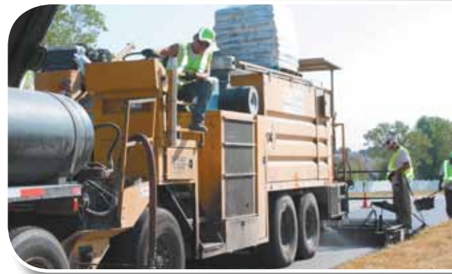
Vance Brothers' Bergkamp continuous mix paver applies micro surfacing made with highly polymer modified asphalt emulsion in Lee's Summit, Mo.
