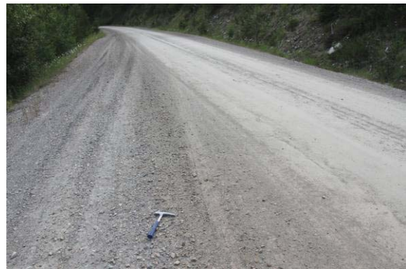
Figure 69. Photo. Untreated shoulder.
