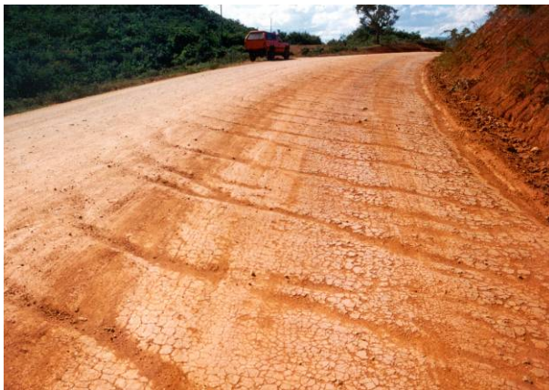
Figure 36. Photo. Transverse erosion.
