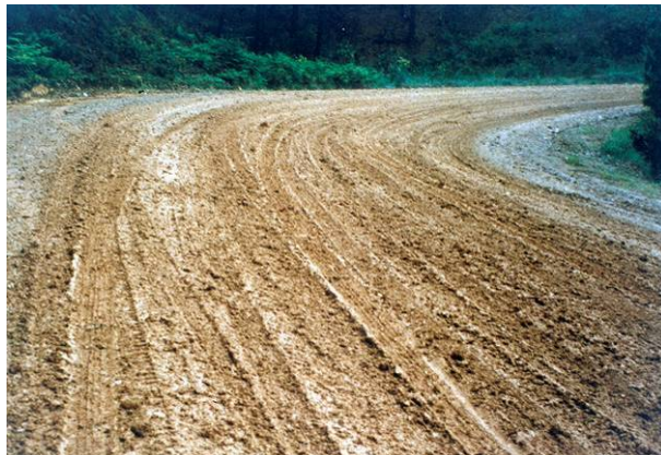
Figure 42. Photo. Slippery when wet.
