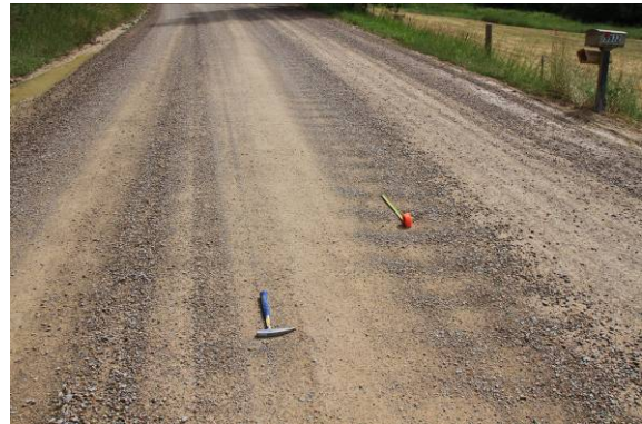
Figure 59. Photo. Chloride applied to poorly prepared road.
