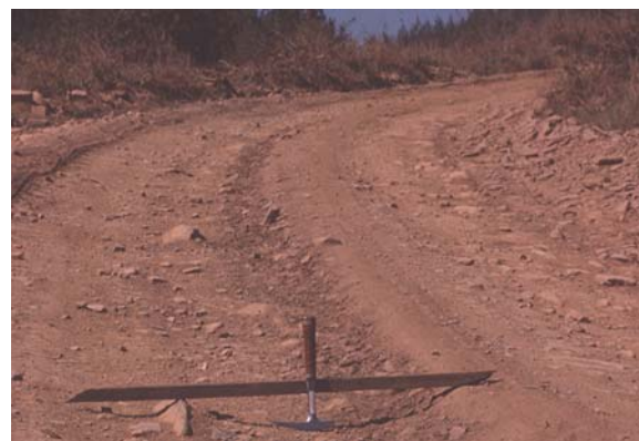
Figure 2. Photo. Poor unpaved road.
