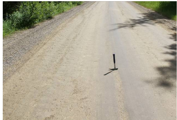
Figure 12. Photo. Crust on road treated with magnesium chloride.
