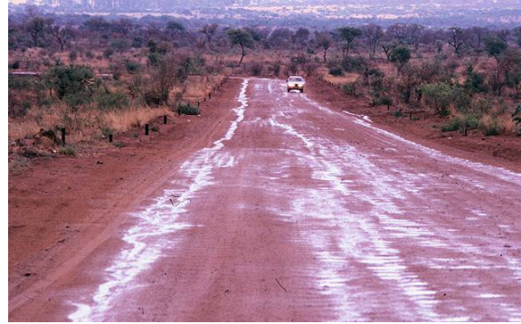
Figure 15. Photo. Excess runoff of chemical treatment.
