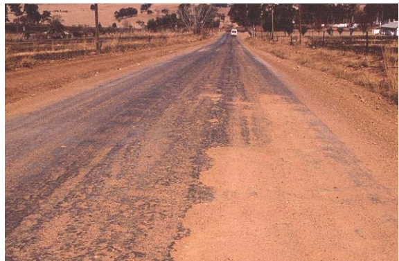
Figure 17. Photo. Broken crust.
