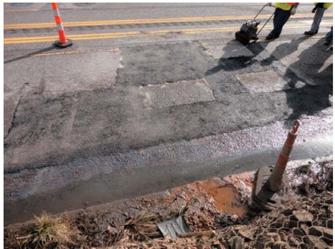
During compaction of patches with plate compactor, water is forced out of the road's subgrade
