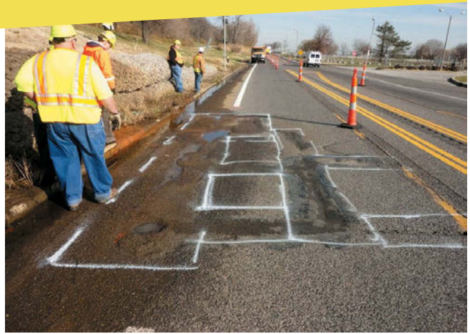
Existing damaged pavement is marked and work zone established prior to patching
