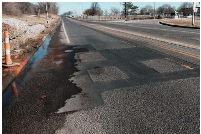
Seven weeks after installation patch is intact, even with water on pavement
