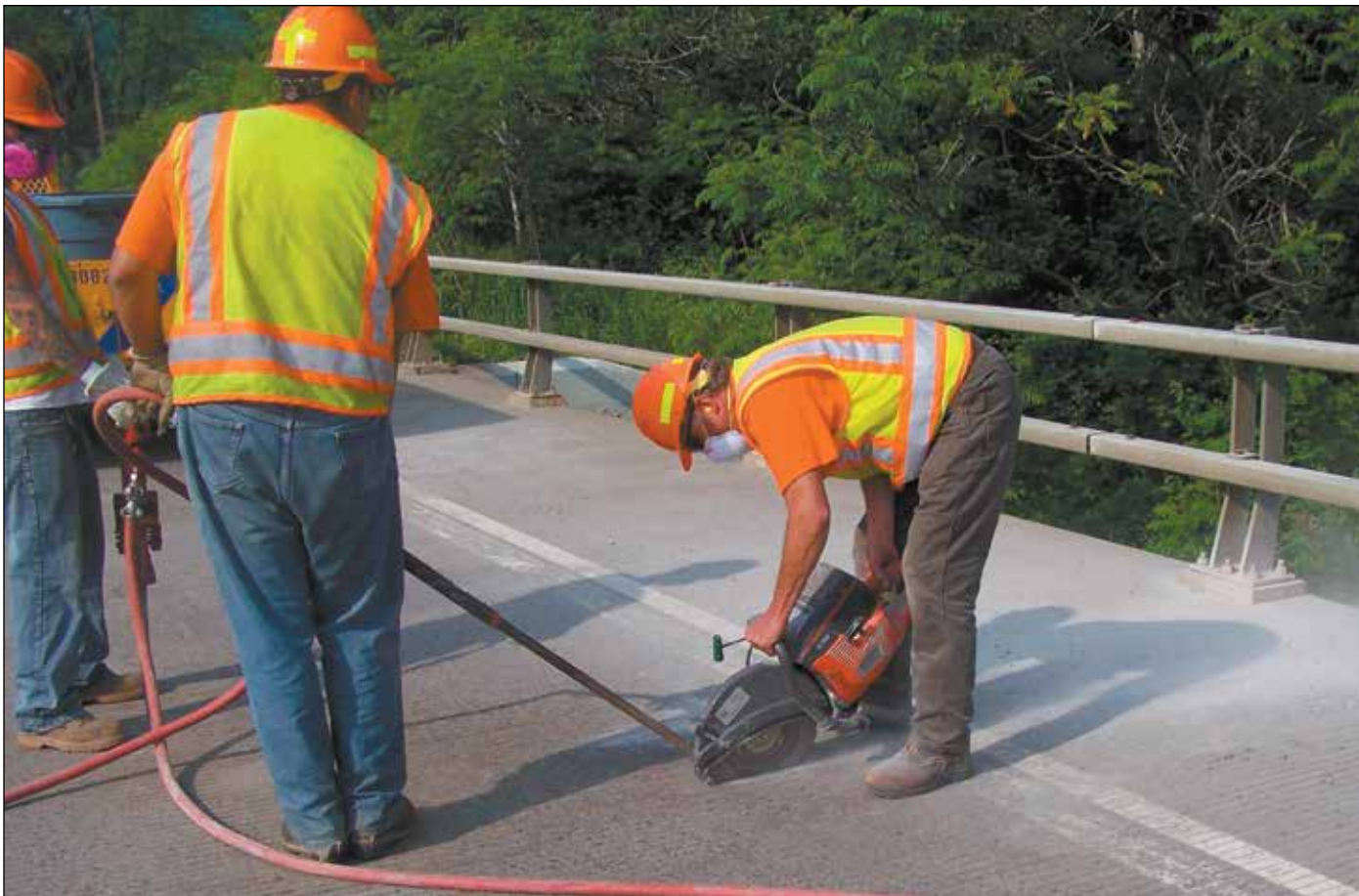
Sawcut is made delineating deteriorated section of concrete deck to be removed for patching demonstration.
