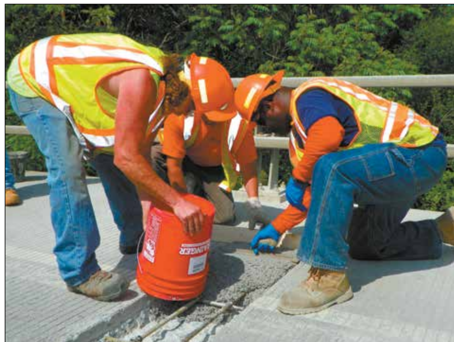
A worker deposits MALP concrete into the repair section as two others screed the fast-setting material.
