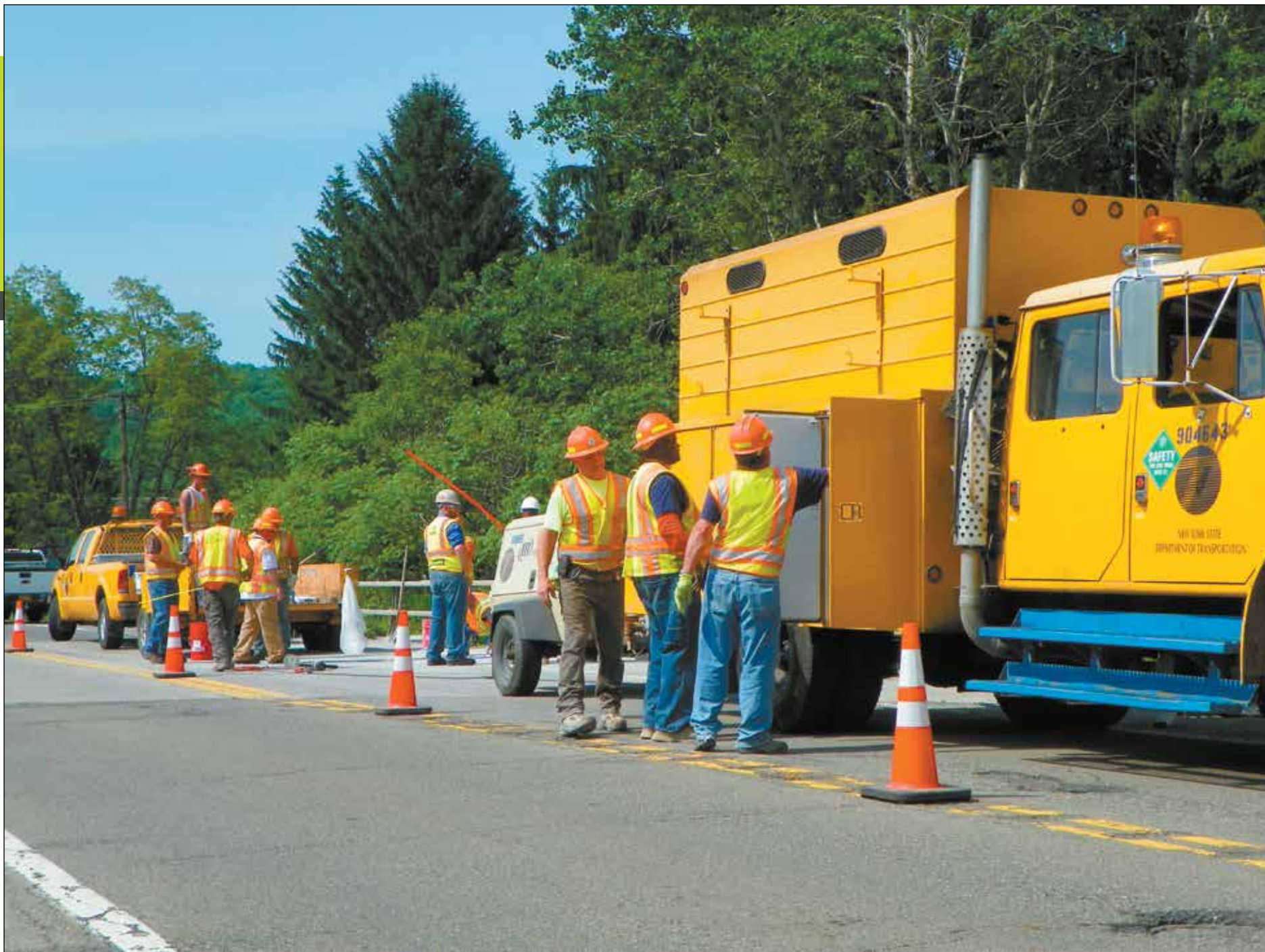
Maintenance crew prepares for demonstration of MALP concrete repair technology on Route 26 bridge over Nanticoke Creek in Maine, New York.
