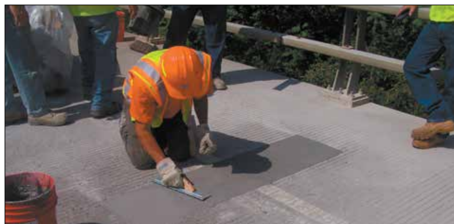
Standard trowels and floats are used to finish the material, which will set up to a compressive strength of 4,000 psi in one hour and more than 7,000 psi in 7 days.
