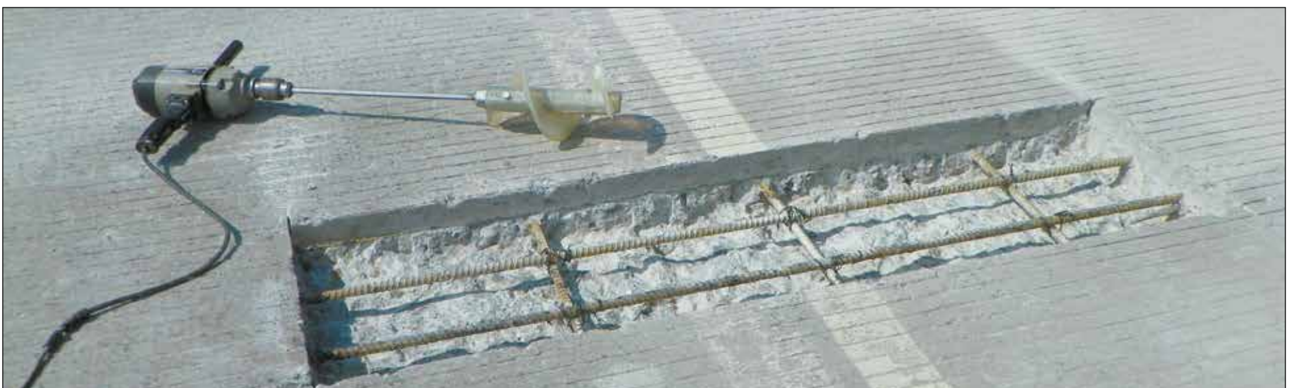
With loose and damaged concrete removed, the section is ready for patching material. Note heavy-duty drill and auger used to mix two patching ingredients.
