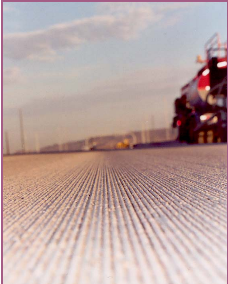
Photo depicts diamond ground pavement. Diamond grinding is used to restore pavement surfaces, remove joint faulting, and improve skid resistance. (Photo: Bill Davenport, ACPA)
