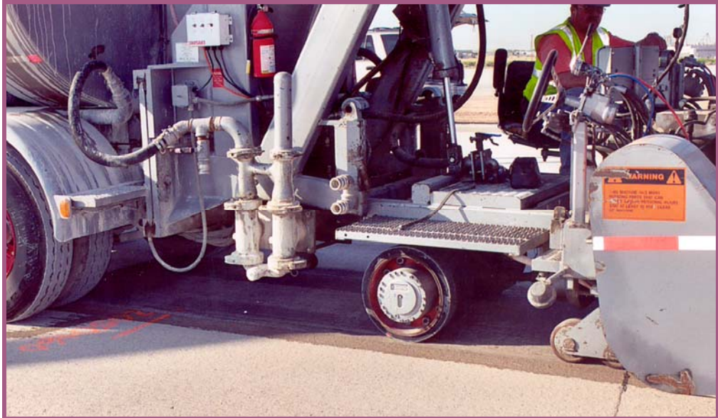
Photo depicts diamond grinding on one of four sections of highway in Arizona. Diamond grinding reduced the tire/pavement noise to 95.5 dbA (using the CPX method). An Arizona DOT report stated: “the use of pavement grinding as a traffic noise abatement could be beneficial for both reducing tire pavement noise levels and muting the tire whine pure tone sound of the older concrete pavement transverse tining texture.” (Photo: Bill Davenport, ACPA)
