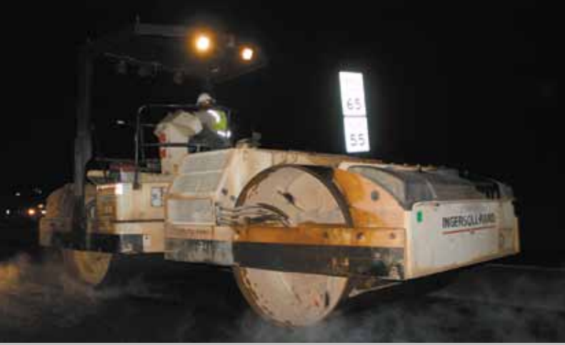
One of two Ingersoll Rand Rollers consolidates the mix for the Interstate 5 demonstration.
