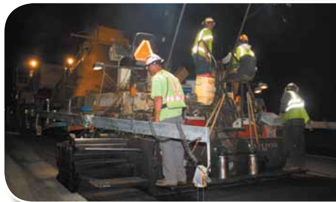
Knife River Materials' Blaw Knox 5510 paver installs thin-lift overlay on Oregon's I-5 near Medford during night demonstration of HiMA for ODOT.
