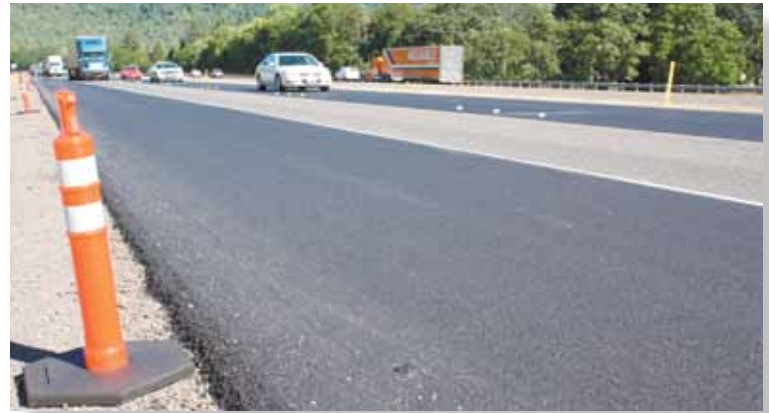
Vehicles travel on I-5 northbound lanes, with HiMA paved shoulder at far left, middle lane with no overlay, and HiMA paved fast lane at right.
