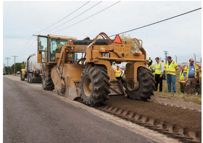
Full-depth recycling using lime slurry is demonstrated by Rock Solid Stabilization & Reclamation with Caterpillar RM 500 stabilizer
