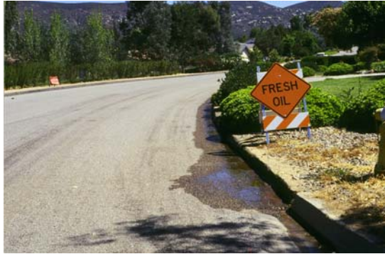
Figure 5-5 Irrigation damage to new chip seal
