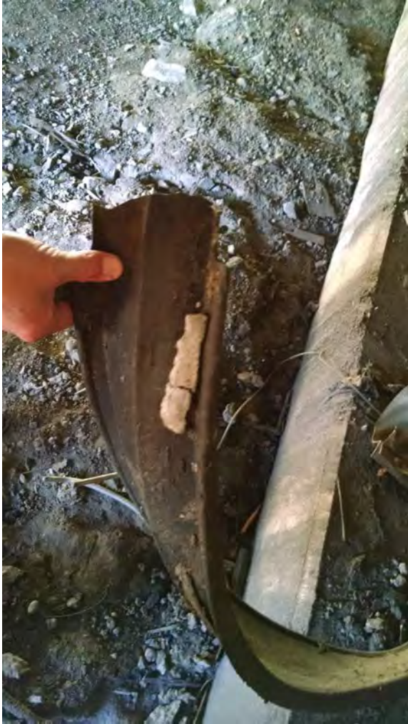
Photo No. 7 – Concrete Adhered to Bottom of Strip Seal Gland (South Abutment Joint)
