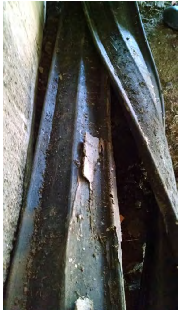
Photo No. 8 – Concrete Adhered to Bottom of Strip Seal Gland (South Abutment Joint)
