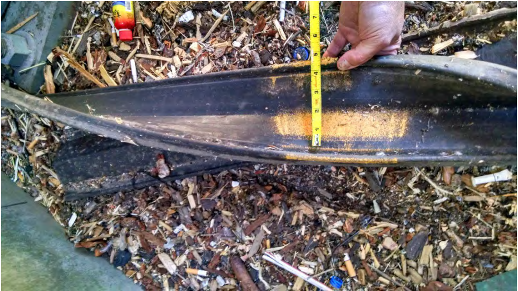
Photo No. 6 – South Abutment Strip Seal Joint Gland w/ Paint on Upper Ears
