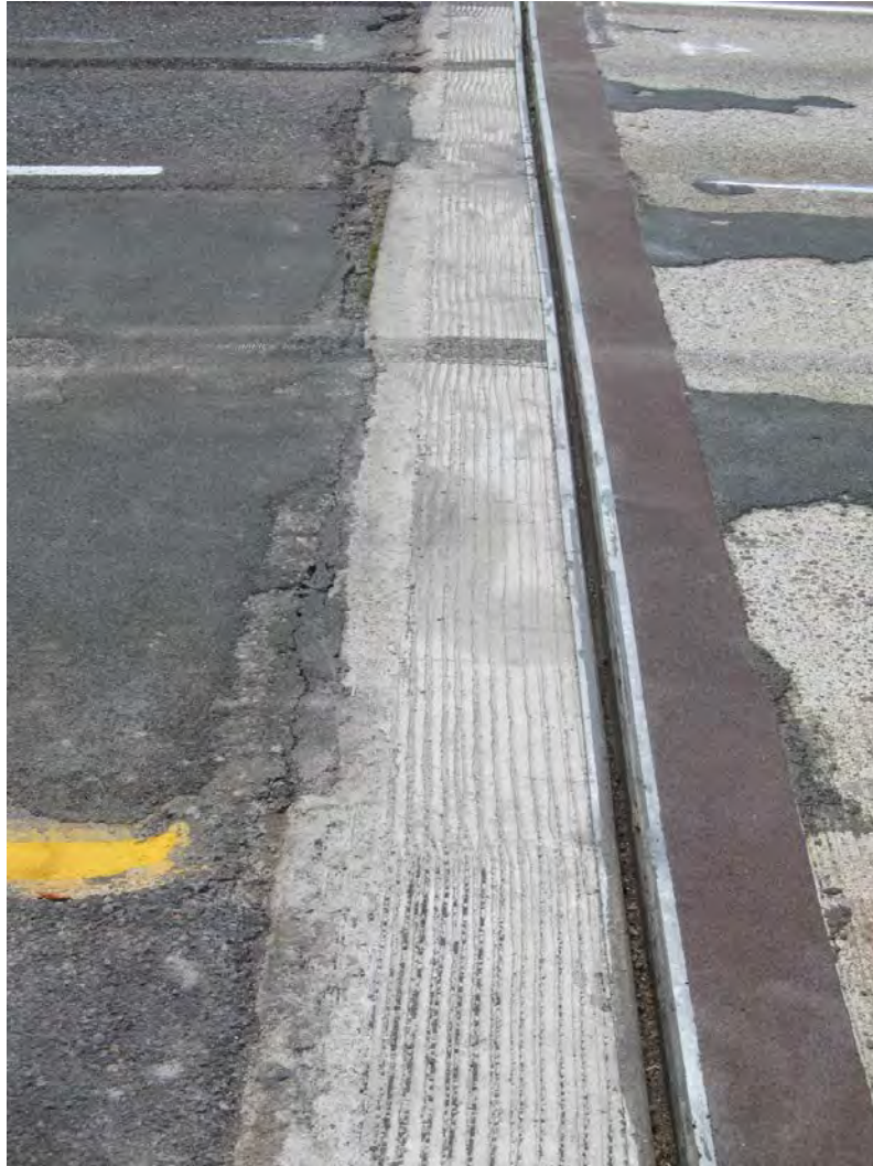
Photo No. 5 – Paint Stripe Removal and Cracks Over Anchorage Plates
