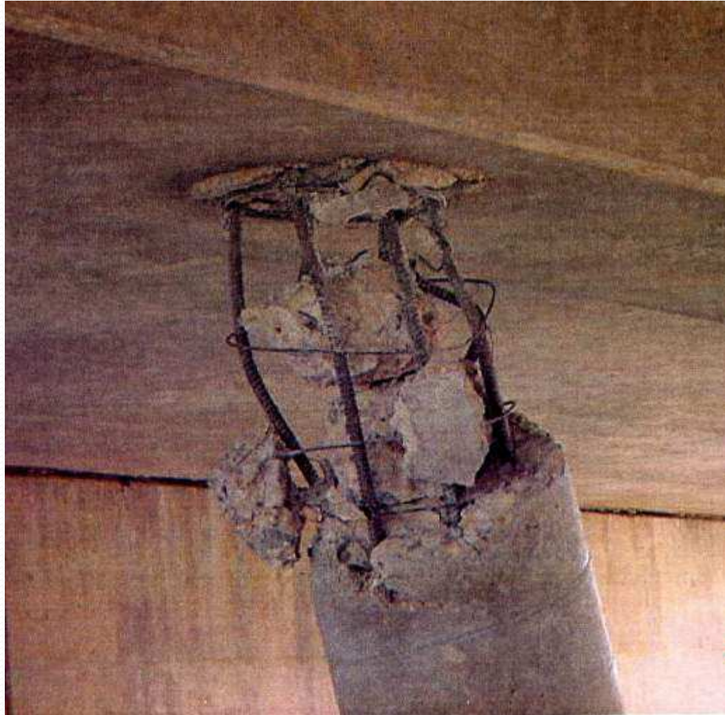
Column 2 bent cap joint failure - typical
