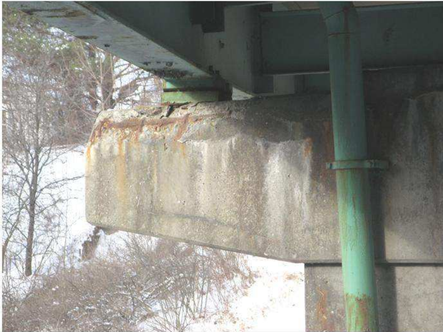
Heavy scaling at east pier cap
