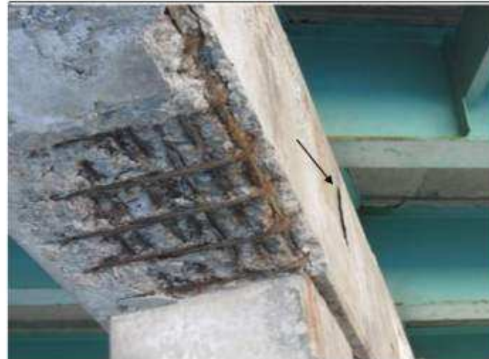
Easterly pier, arrow denotes impending spall.
