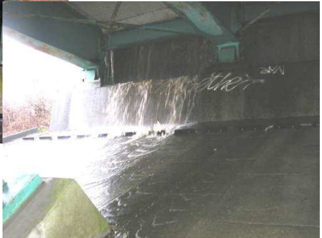
Failed deck joint during rain storm
