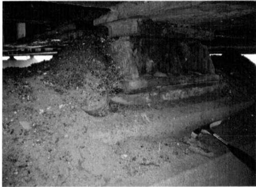
Photo # 26: Typical condition of bearings at pier 9 with heavy laminated rust, up to ¼ inch loss on rockers and masonry plate and heavily covered with bituminous concrete.
